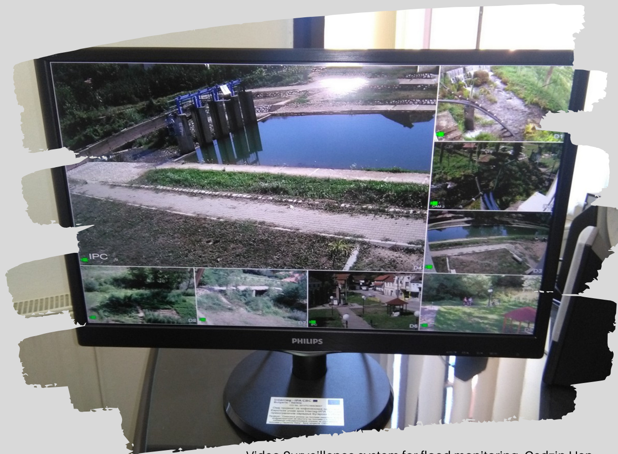
Video Surveillance system for flood monitoring, Gadzin Han
